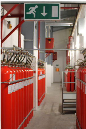
Fire protection in our site
