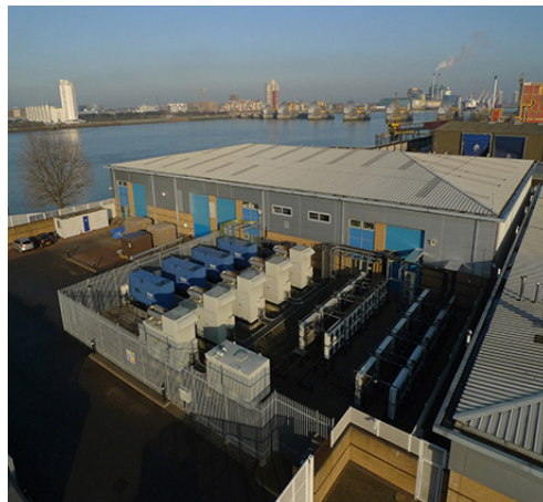
Aerial view of Six Degrees' London Data Centre
